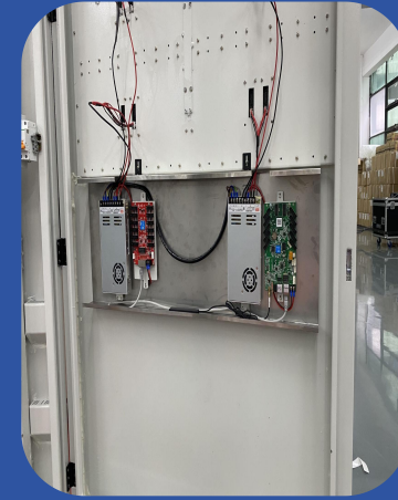
Power Supply and Control system
